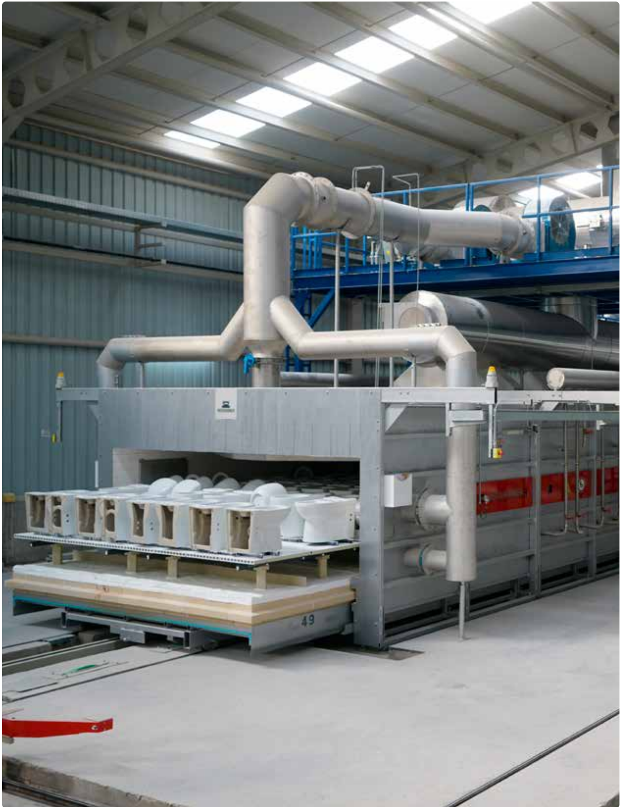
TUNNEL KILN with cars, complete with car circulation system
