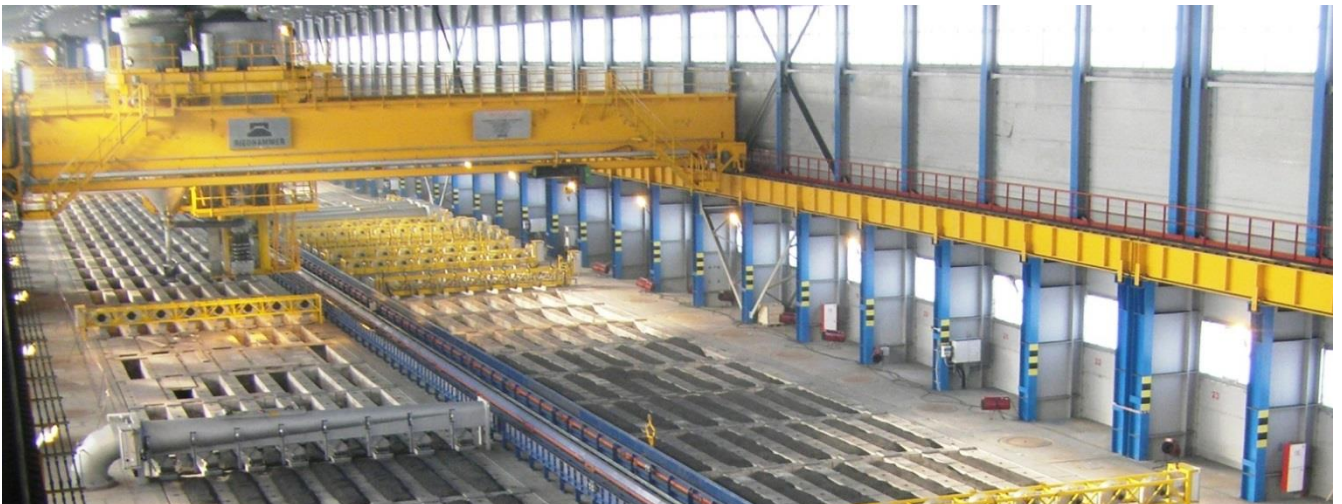
Open Top Anode Baking Furnace
