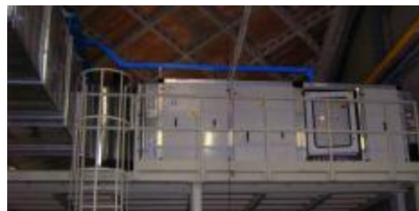
Air treatment unit
