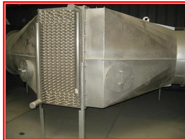
Shell and tube heat exchanger (Flue Gas / Water)
