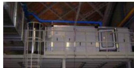
Air treatment unit
